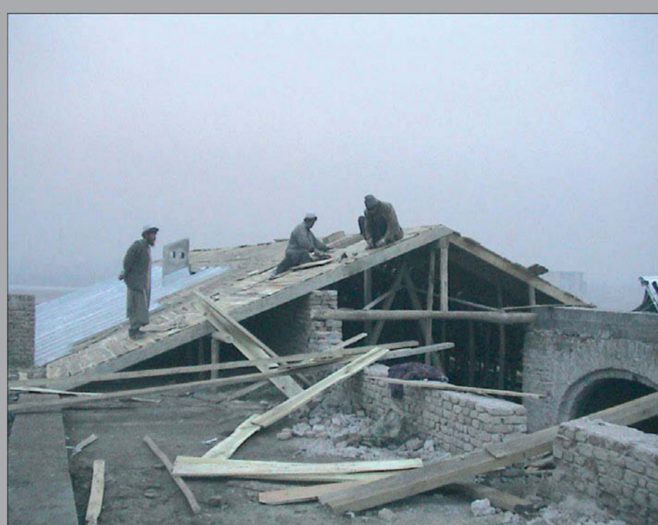
Repairing the roof of the National Museum. Photo by Ana Rodriguez 2004/ SPACH Photocatalogue
